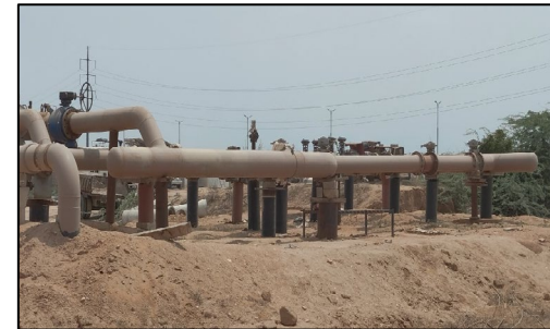
SSGC TBS to provide 13MMCFD RLNG
